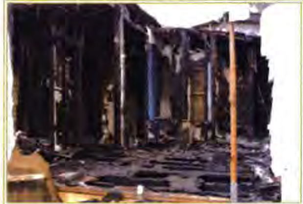
The back half of a residence on Herald Road sits gutted after a fire ravaged the back of the house.
