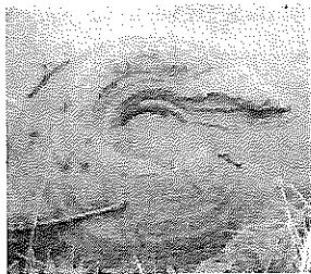
Boil in North Drain near Sacramento River levee
